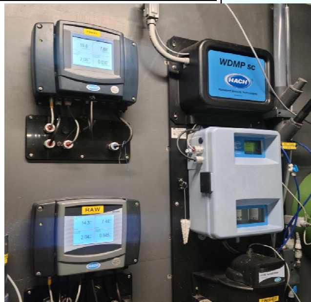
The picture at left shows some of the equipment used to monitor and analyze the water in the treatment plant. This equipment measures chlorine, turbidity, pH and temperature in both the raw and finished water.
